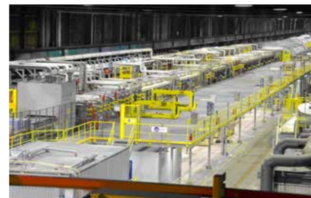
▲ Stainless Steel CAPL at Outokumpu, Finland
