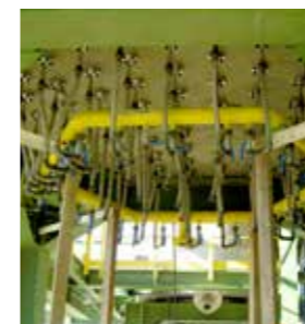
▲ Burners situated on the reactor bottom - Fluidized Bed ARP
